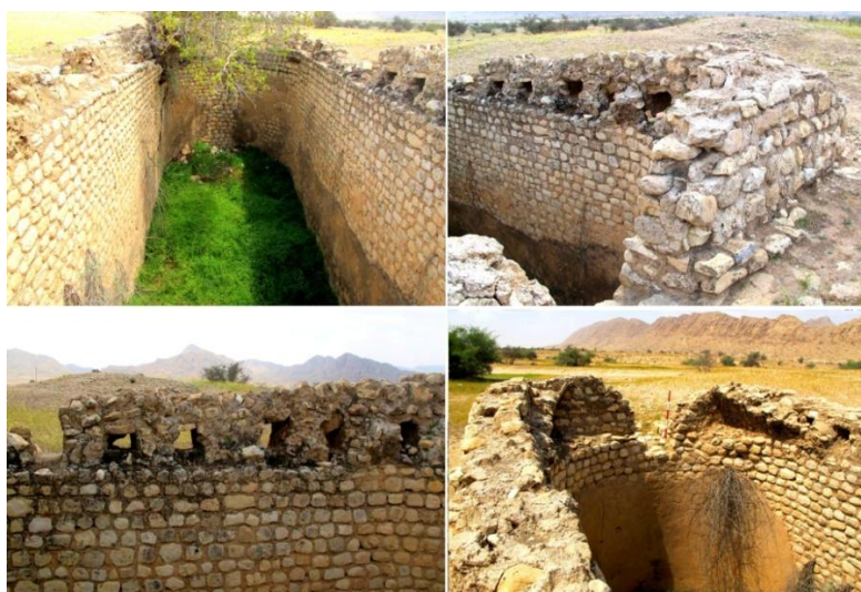
Fig 18: Input doors, windows, and the arches of destruction on the pool (Photo by: Writer)
