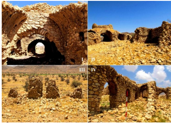
Fig 14: I: Room IV; II: Room II, IV, VII; III: part of wall destruction out the series the south eastern side; IV: Hall A (Photo by: Writer)
